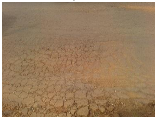
Plate 2. Failures at CH. 0+000 – 0+500
